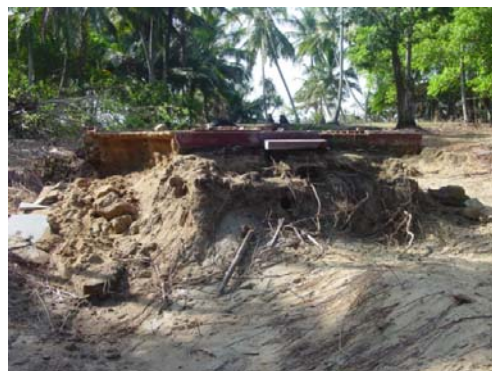
Completely destroyed house in the beach front
